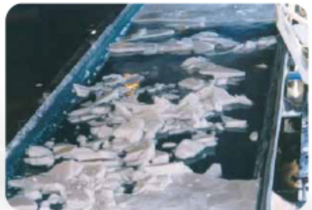
FZ-5: CONVEYING CAUSTIC SODA
